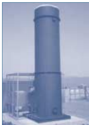
Figure 2.5 A typical enclosed flare
