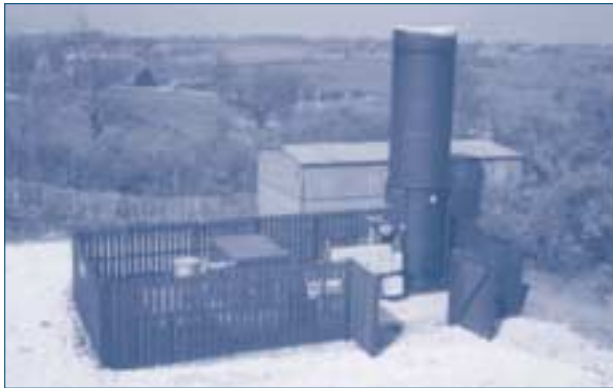
Figure 4.3 | Enclosed flare station
