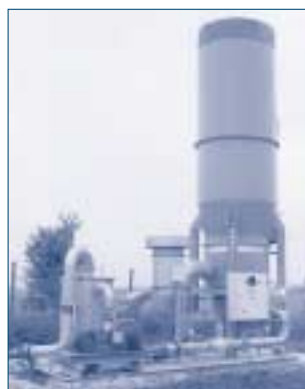
Figure 2.6 | Example of a forced air enclosed flare
